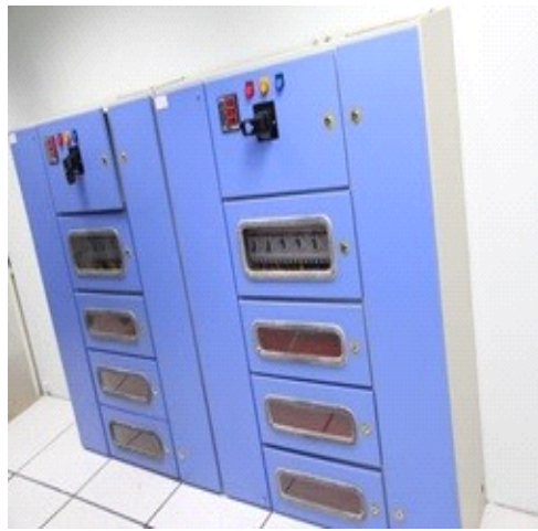
Figure 7: Power Distribution Unit (PDU)
